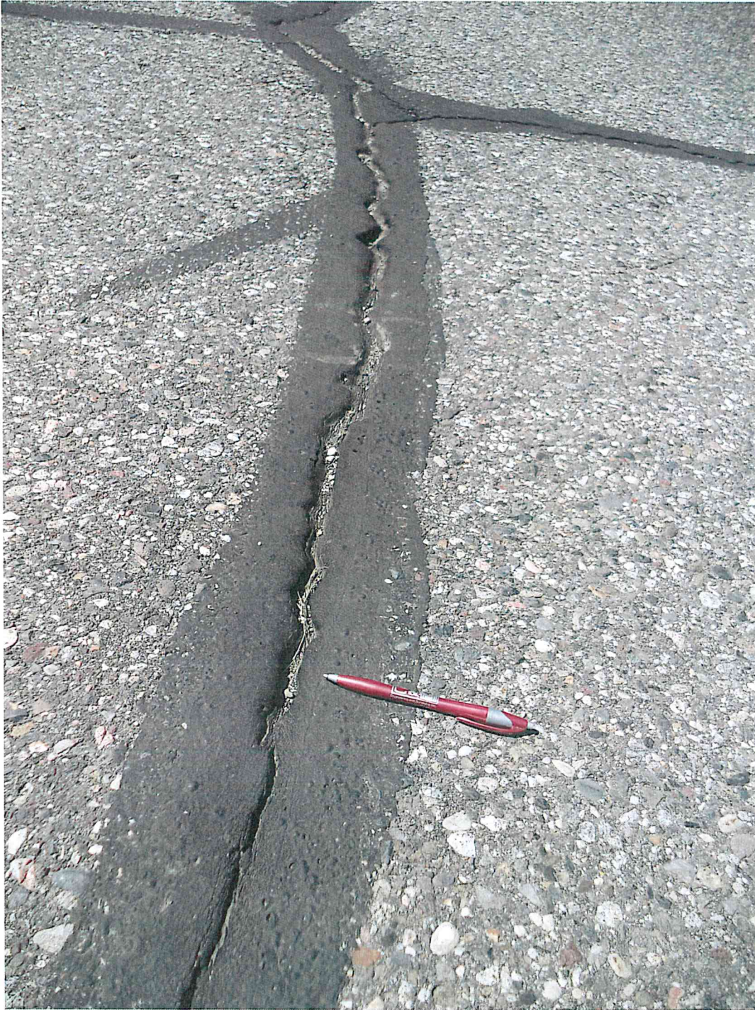
Picture 1 - typical patched crack
